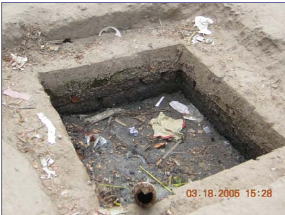
Photo - 3.22. Open manhole in Jatrabari area
